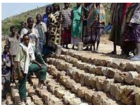
Sediment storage dams under construction (Ethiopia) Daniel Danano, NR for Ethiopia ethiocat@ethionet.et
