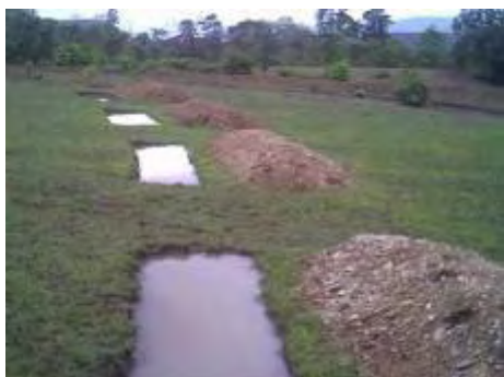
Staggered contour trench for water and soil conservation (India) G.B. Reddy, Orissa Watershed Development Mission, India bhaskar_gala@yahoo.com
