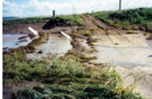
concrete (in previous floods, without vetiver protection the crossing was destroyed and had to be rebuilt. Photo by Paul Truong
